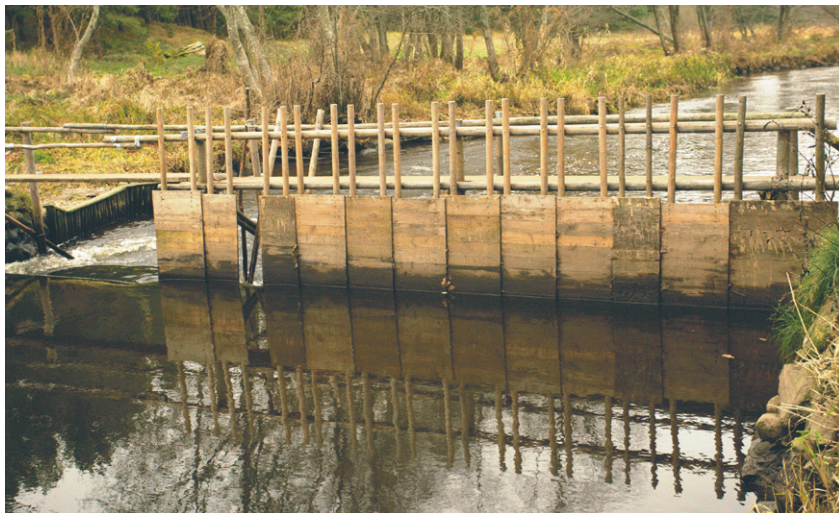
Fig. 83. The same weir as in Fig. 82, but in 2011 with lower water levels. The construction of the wooden barrier can be clearly seen, as well as the opening in the barrier where mesh gear with a lifting frame is placed on the other side of the barrier. 8 November 2011. Photo: Kjell Sjöberg.
